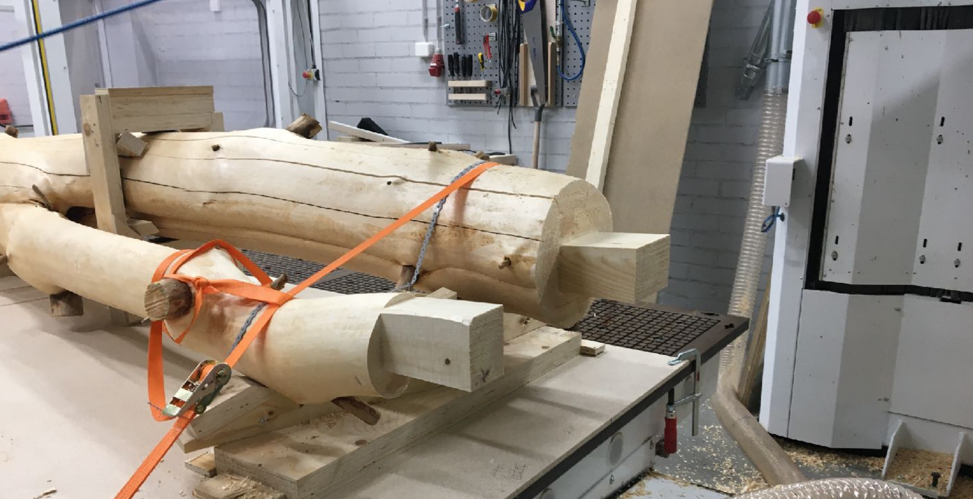
Roof connections, fabricated with a 5-axis NC router. Aalto University Wood Program, 05/2020.
